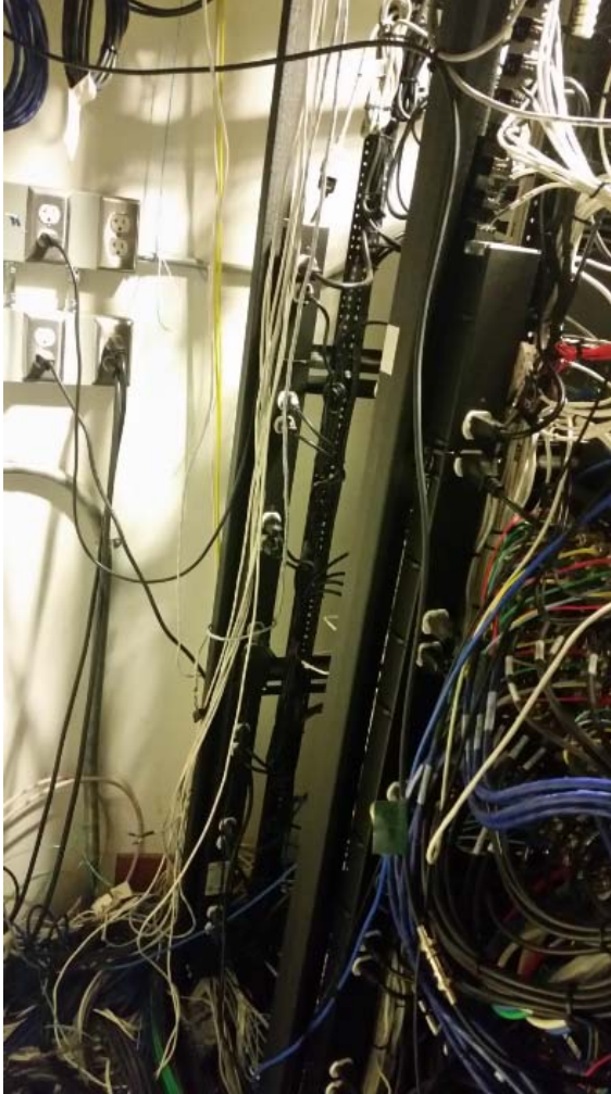
Picture 4- Audiovisual Rack Cabling
